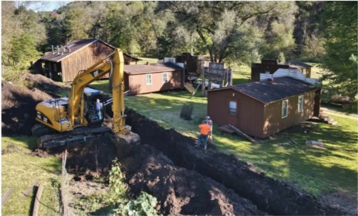
New water lines to the dining hall were constructed to accommodate Sugar Creek's new guests, and this work was cost-shared with the farm at 50%.
