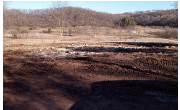
More soil is needed here to fully bury and cover the house's foundation.
