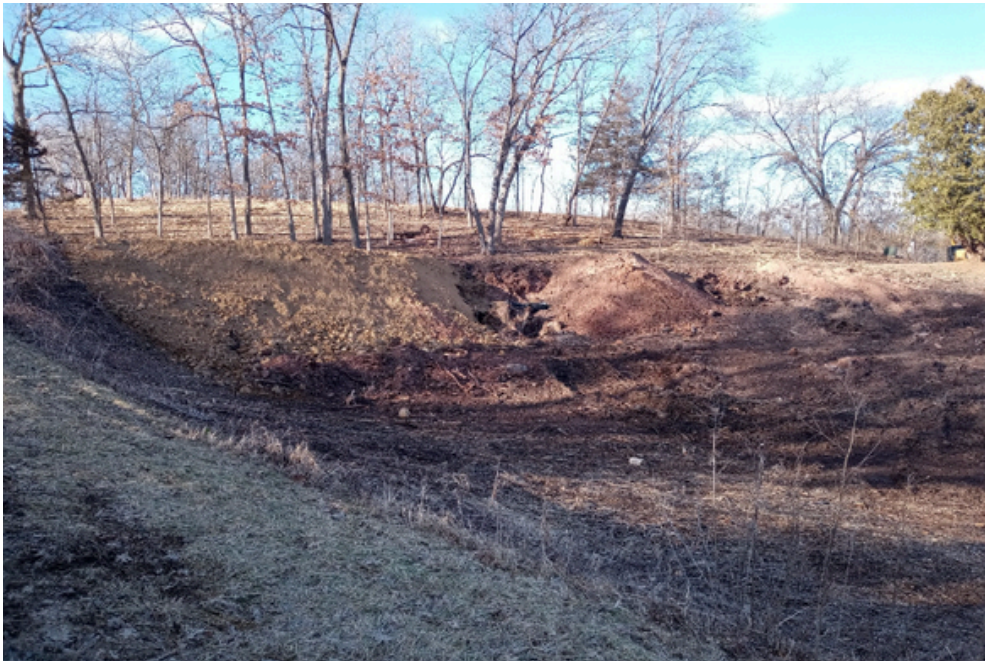
More loads will be needed, here, along the edge of the driveway.
